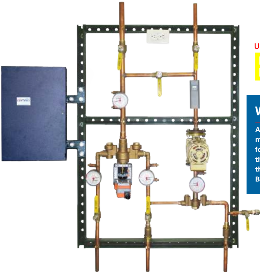
COMMAND STATION UPGRADED WITH BASyC
